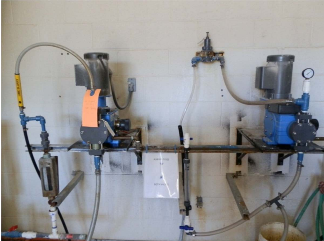
Figure 5-11 Lime Feed Pumps
