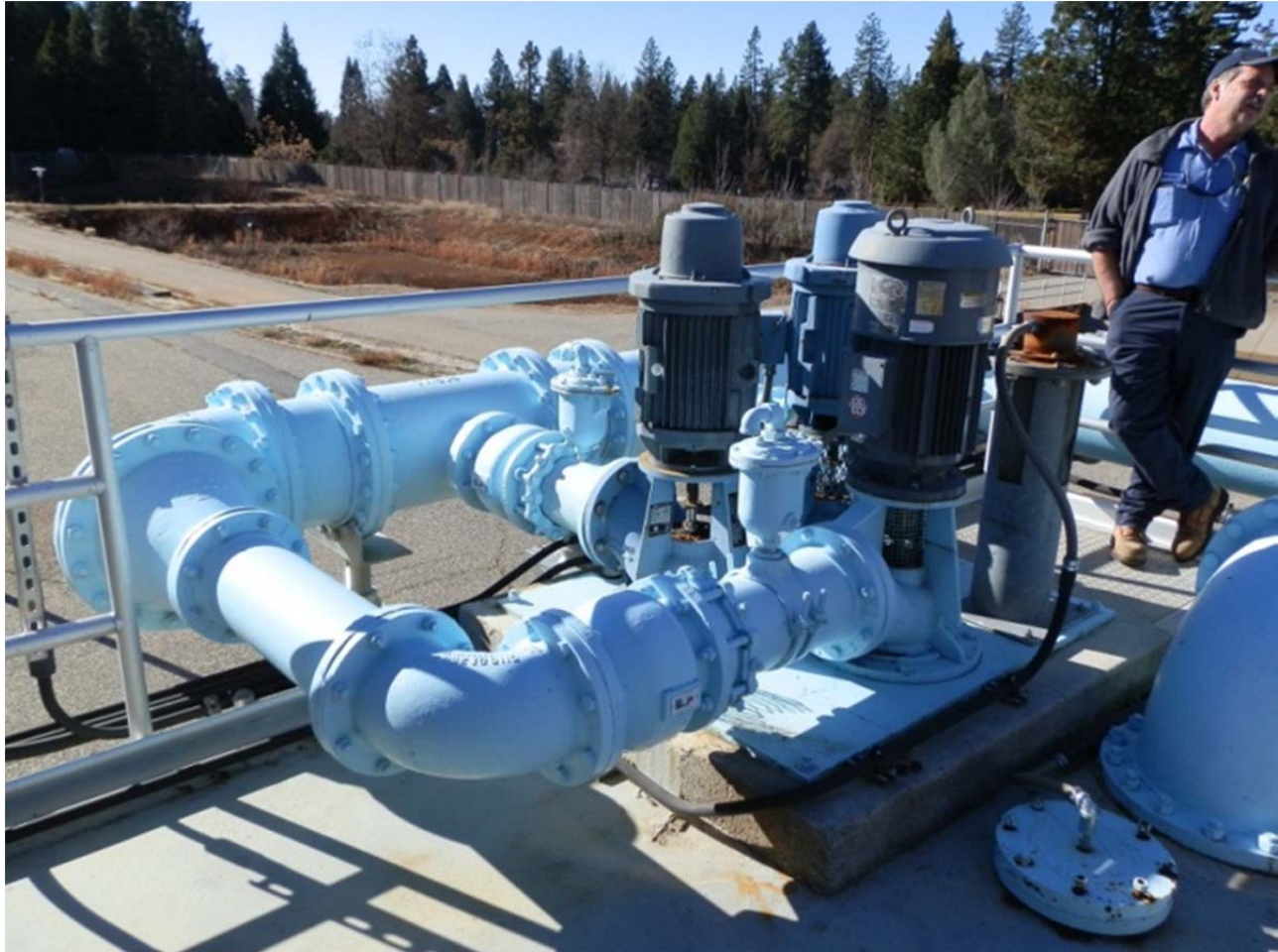
Figure 5-9 Filter Backwash Pumps
