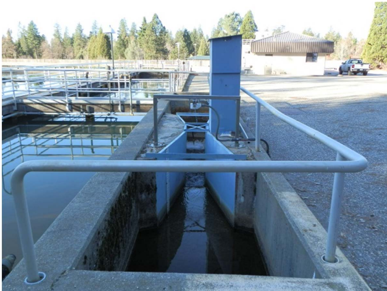
Figure 5-3 Parshall Flume in Raw Water Inlet Structure
