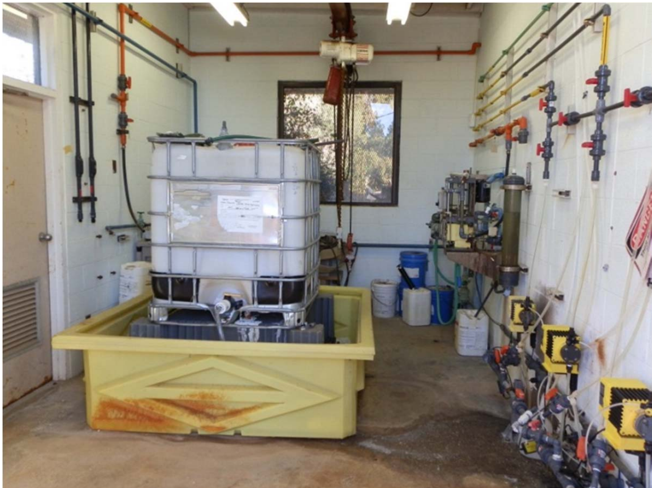
Figure 5-10 Polymer Storage and Sodium Hypochlorite Feed Pumps – Chemical Feed Building
