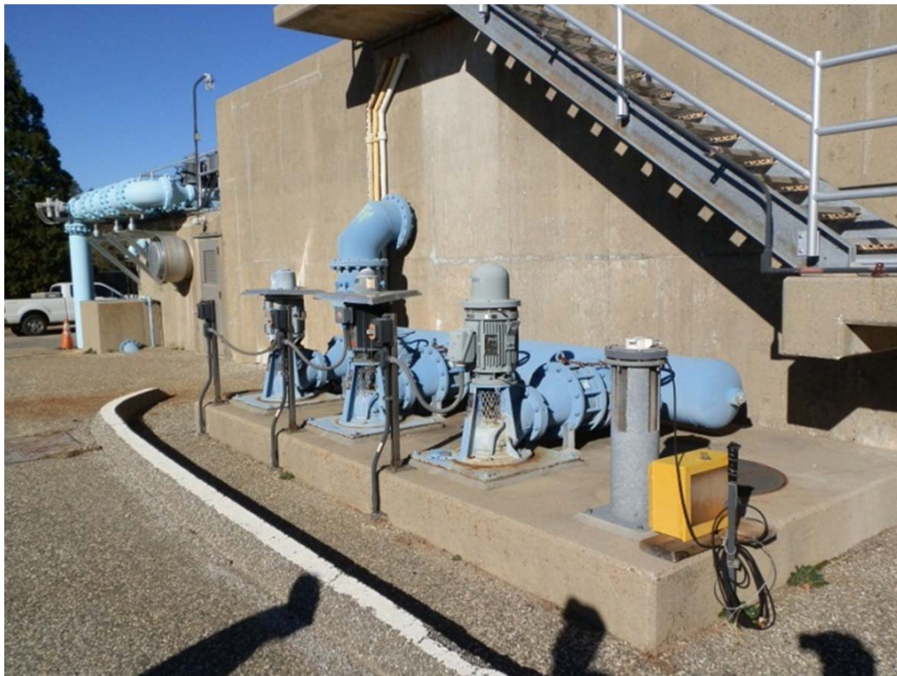
Figure 5-7 Vertical Turbine Filter Supply Pumps
