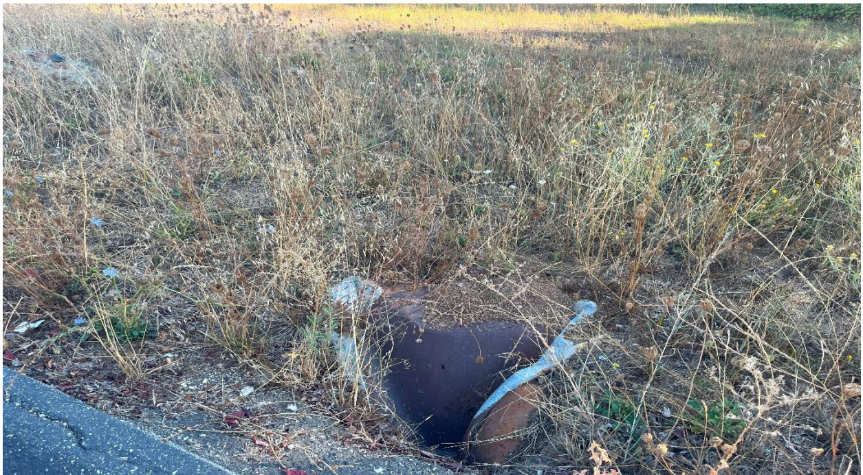
Photo 8: Existing culverted drain to the east of the Lumberjack's back parking area. The drainage within the site leaves in culverts and ends up underground within the City's stormwater management system before daylighting at Olympia Creek to the south.
